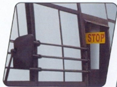
Window railings for safety
